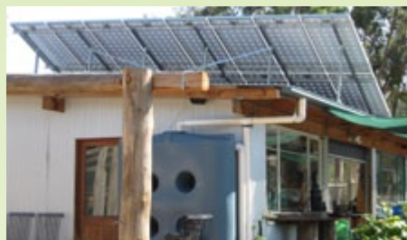
A 4 Kilowatt Solar System at the Wandella production site (one of two Solar Systems).
